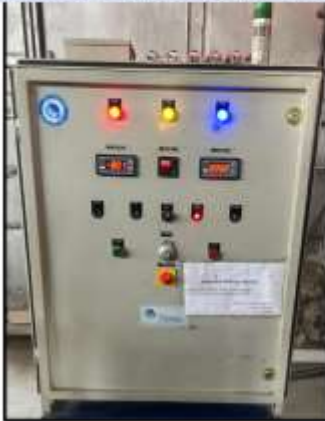
Induction Melting Furnace
